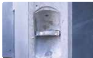
No concrete in the hole!
